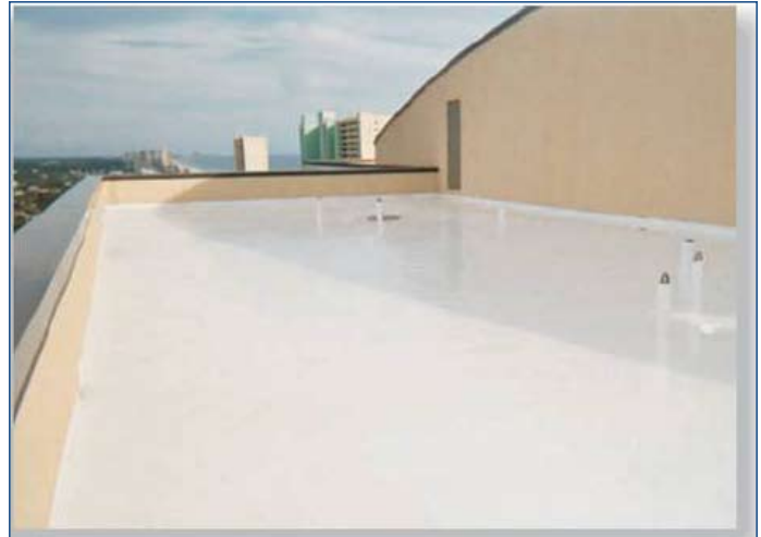
The Vulkem® 360NF/951NF Deck Coating System on this condominium rooftop at the Origins of Seahaven in Panama City Beach, Florida meets Energy Star™ requirements for reflectivity and emissivity and contains minimal VOCs.
