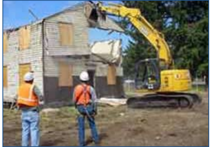
World War II era buildings being "deconstructed" in order to increase the recovery of useable materials
