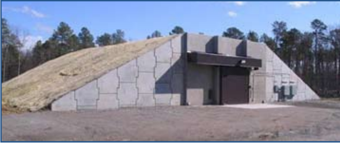
Construction of the first of five munitions supply buildings to securely store small arms, Fort Lee VA
